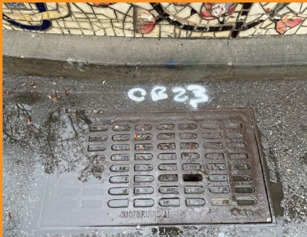
Example: Unmanaged sediment clogging catch basin grates.
