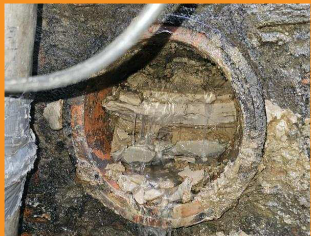
Example: Unmanaged concrete washout clogging pipes.
