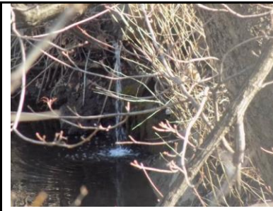
Dry weather discharge observed exiting storm sewer outfall HP-650 from activities in Westchester County in March 2025
