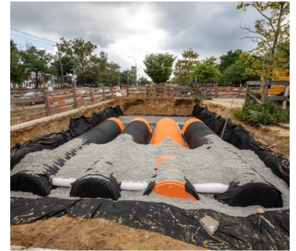
Subsurface water detention
