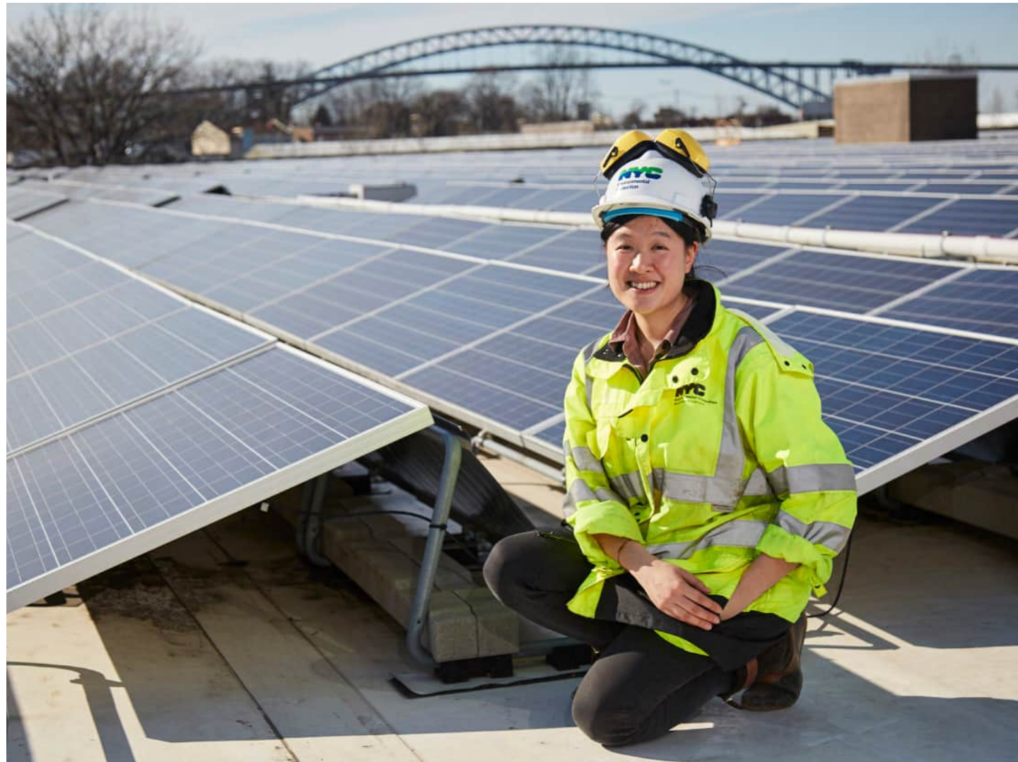
The solar array at the Port Richmond WRRF on Staten Island has been in operation since 2015. Another more expansive installation is being planned at the Wards Island WRRF, including over process tanks. (Courtesy of NYCDEP)
