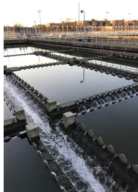
Upgrading critical WRRF infrastructure while maintaining operations is a major challenge for DEP. (Courtesy of NYCDEP)
