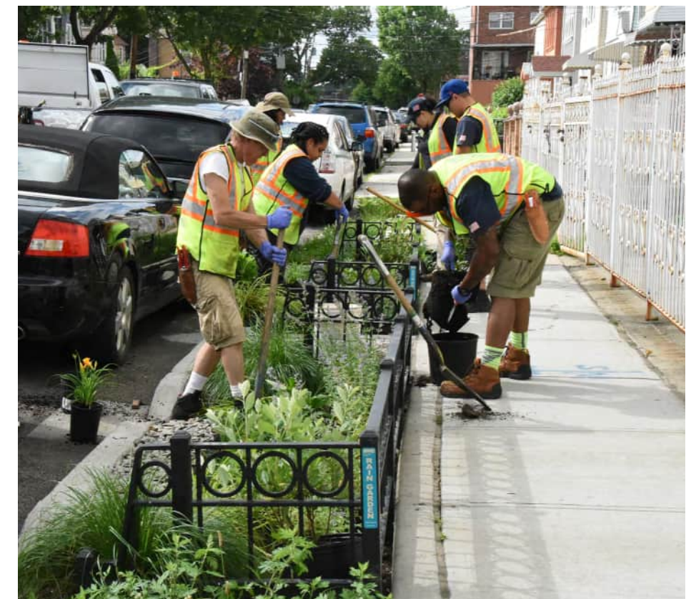
DEP has installed more than 12,000 rain gardens throughout NYC to reduce CSOs, reduce ponding, provide summer shade, and green communities. These features created new green jobs for the City, as DEP hires staff to help maintain them. (Courtesy of NYCDEP)
