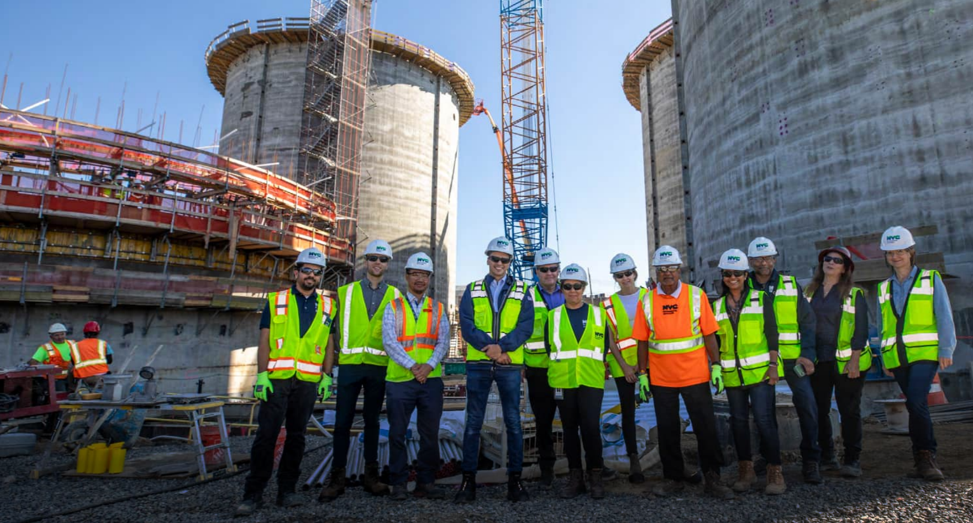
DEP staff working on a digester upgrade project at the Hunts Point WRRF. (Courtesy of NYCDEP)
