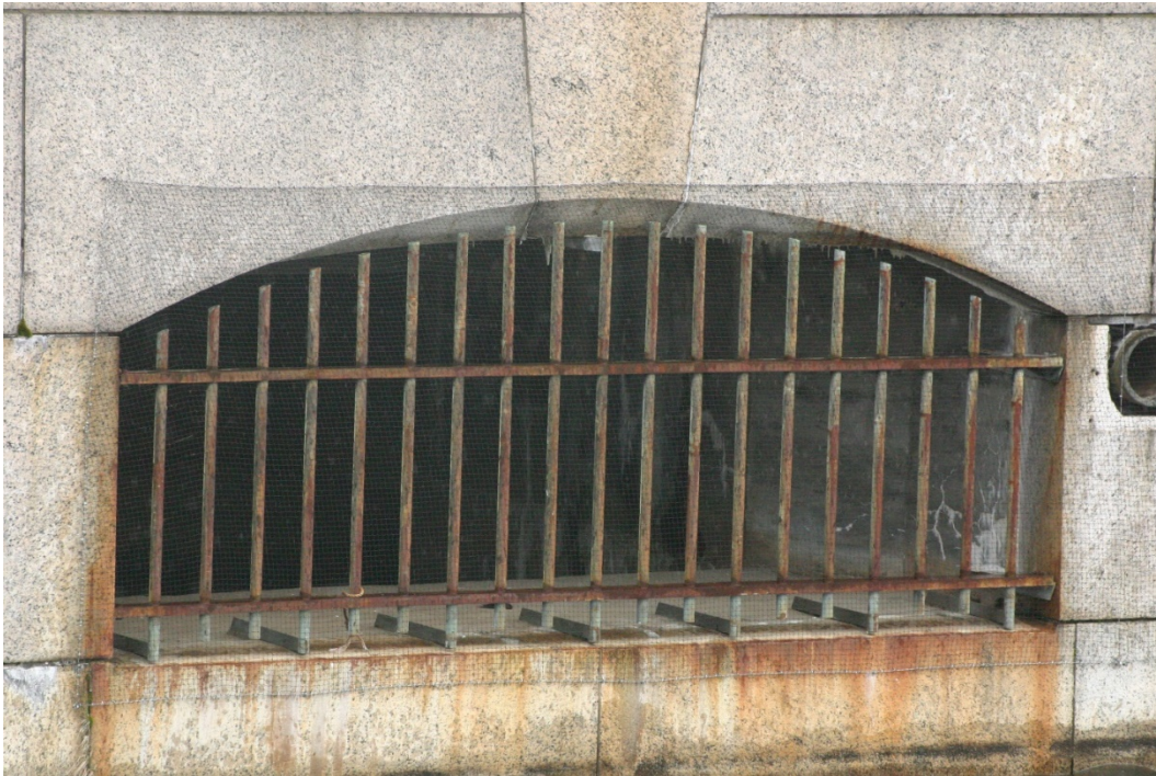
Figure 3.15. Bird deterrent netting maintained on the waterside of Shaft 18 at Kensico to prevent swallows, pigeons, and sparrows from nesting inside the structure. Photo by Chris Nadareski
