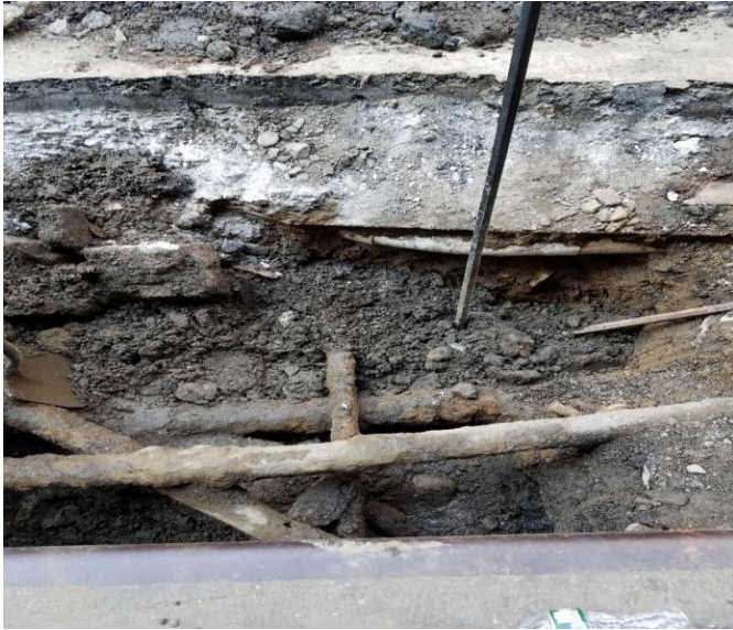
Electrical & wastewater infrastructure
