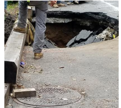
Street systems and underground drainage problems. Photo by R. Zimmerman
