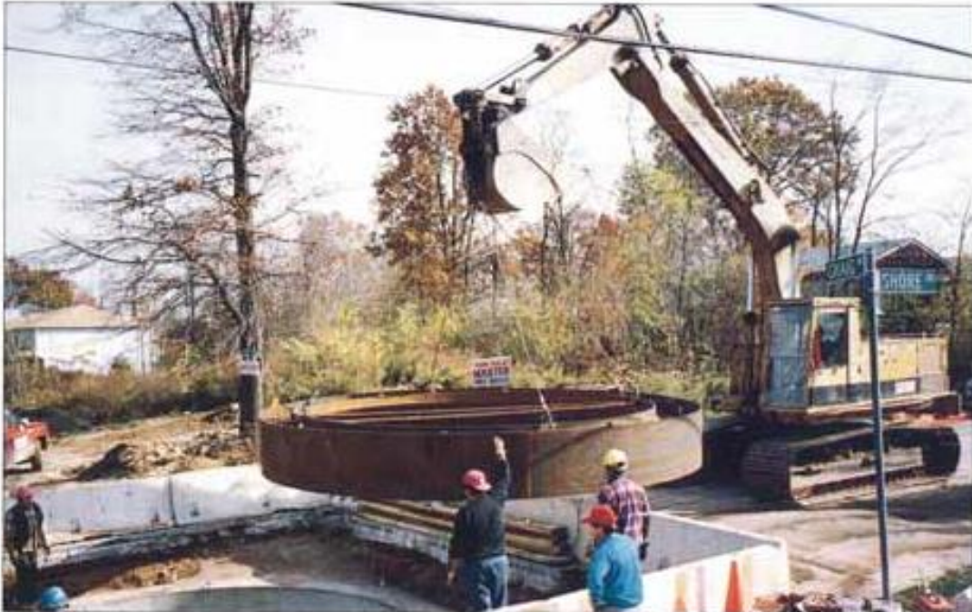
A STEEL CUTTING SHOE IS LOWERED INTO THE STARTING COLLAR OF A MANHOLE SHAFT IN STATEN ISLAND, N.Y. THE SHOE WILL HELP THE SHAFT SECTIONS SET ON TOP OF IT SETTLE INTO THE GROUND.
