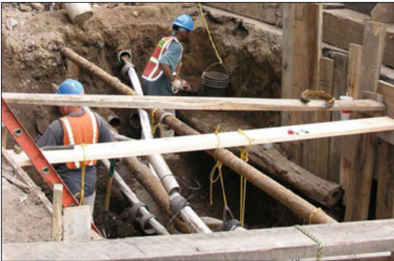
Fig. 1. Wooden water pipes discovered in 2006 during routine utility upgrades in Lower Manhattan [8].
