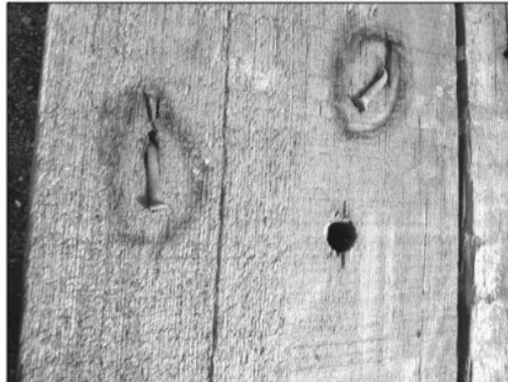
Figure 5. Typical fasteners encountered in reclaimed dimensional lumber, including nails and spikes remaining from prior construction. These fasteners contribute to localized defects, grading reductions, and processing challenges, underscoring the importance of thorough inspection and de-nailing prior to reuse.
