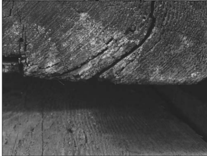
Figure 6. Example of edge decay and fiber separation in reclaimed lumber resulting from prolonged environmental exposure and prior loading conditions. While surface deterioration is evident, such damage is often localized, reinforcing the need to distinguish superficial degradation from core structural integrity.
