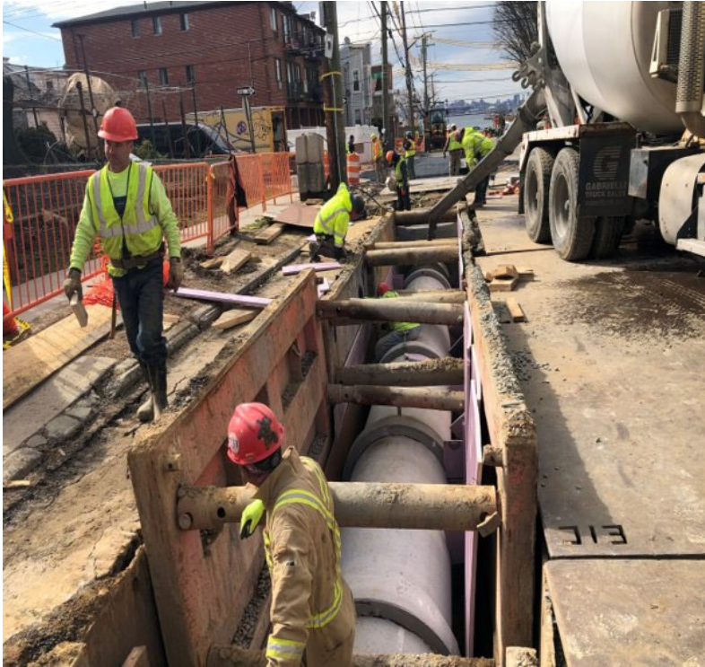
36 inch diameter storm sewer 20 th Avenue between 120 th & 121 st Streets
