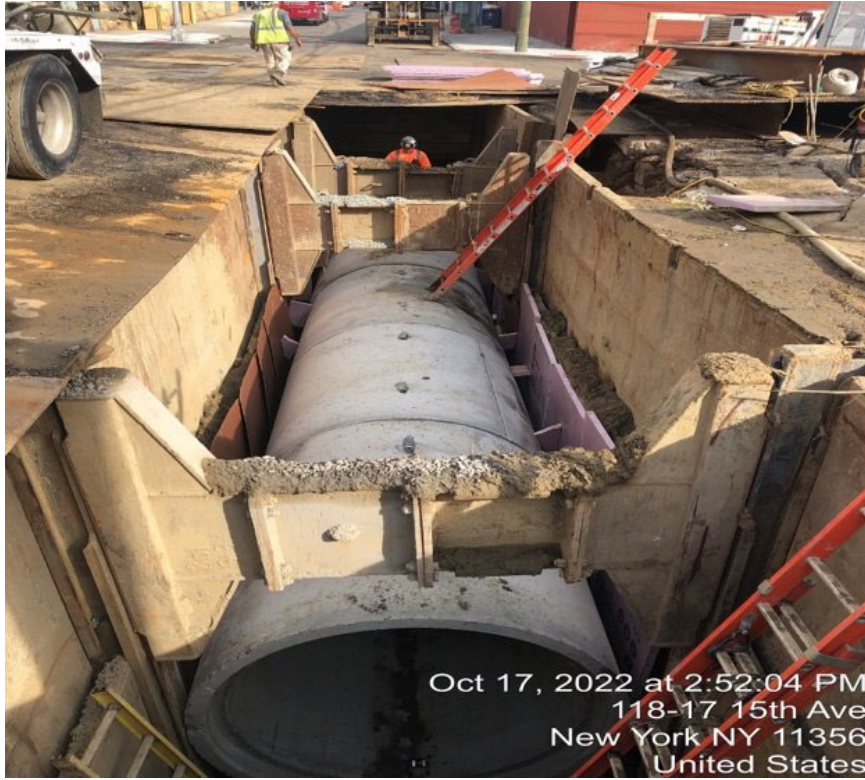
72 inch diameter storm sewer 15 th Avenue between 118 th & 119 th Streets
