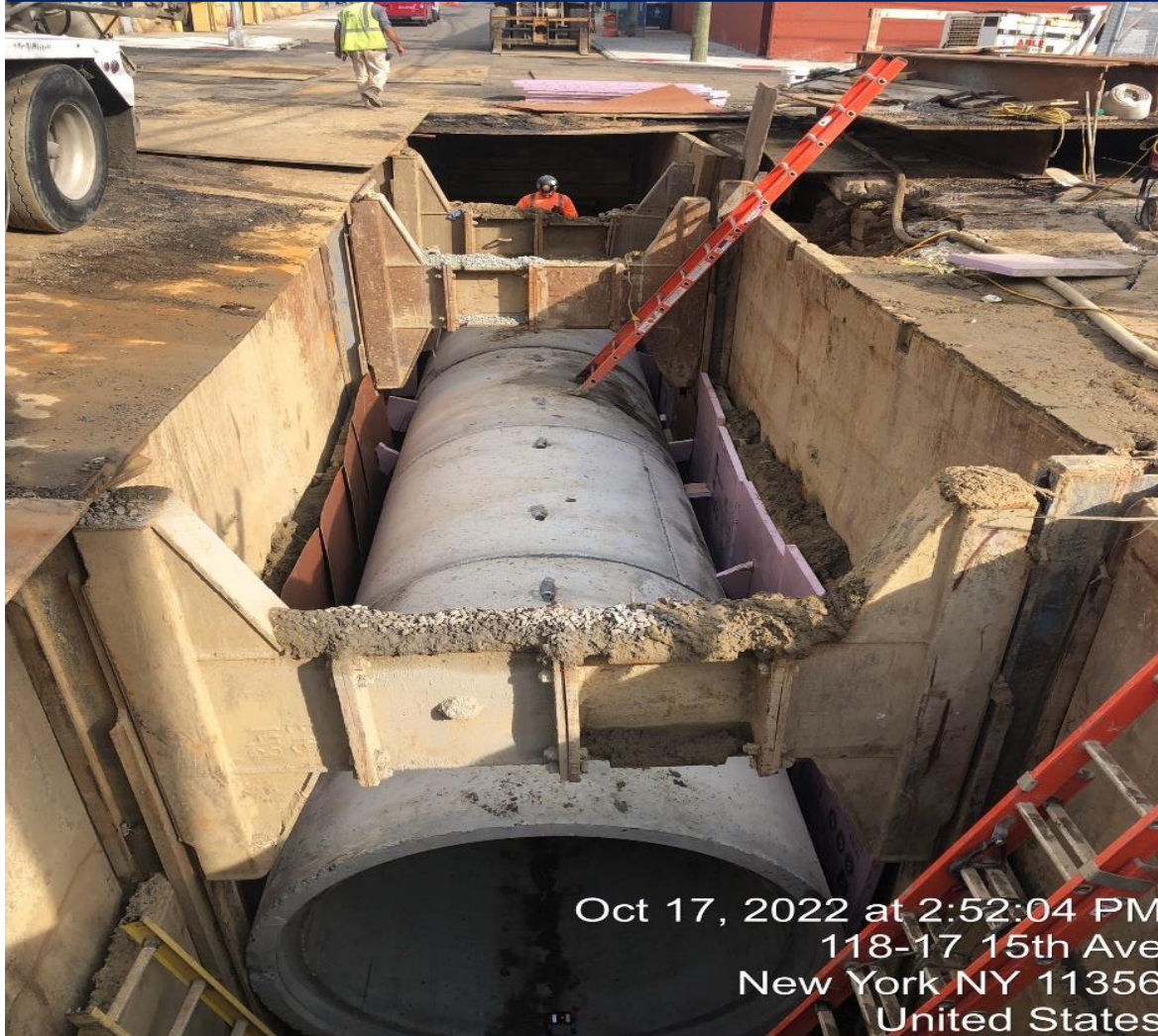
72" dia. RCP Storm Sewer 15 th Avenue between 119 th Street and 118 th Street
