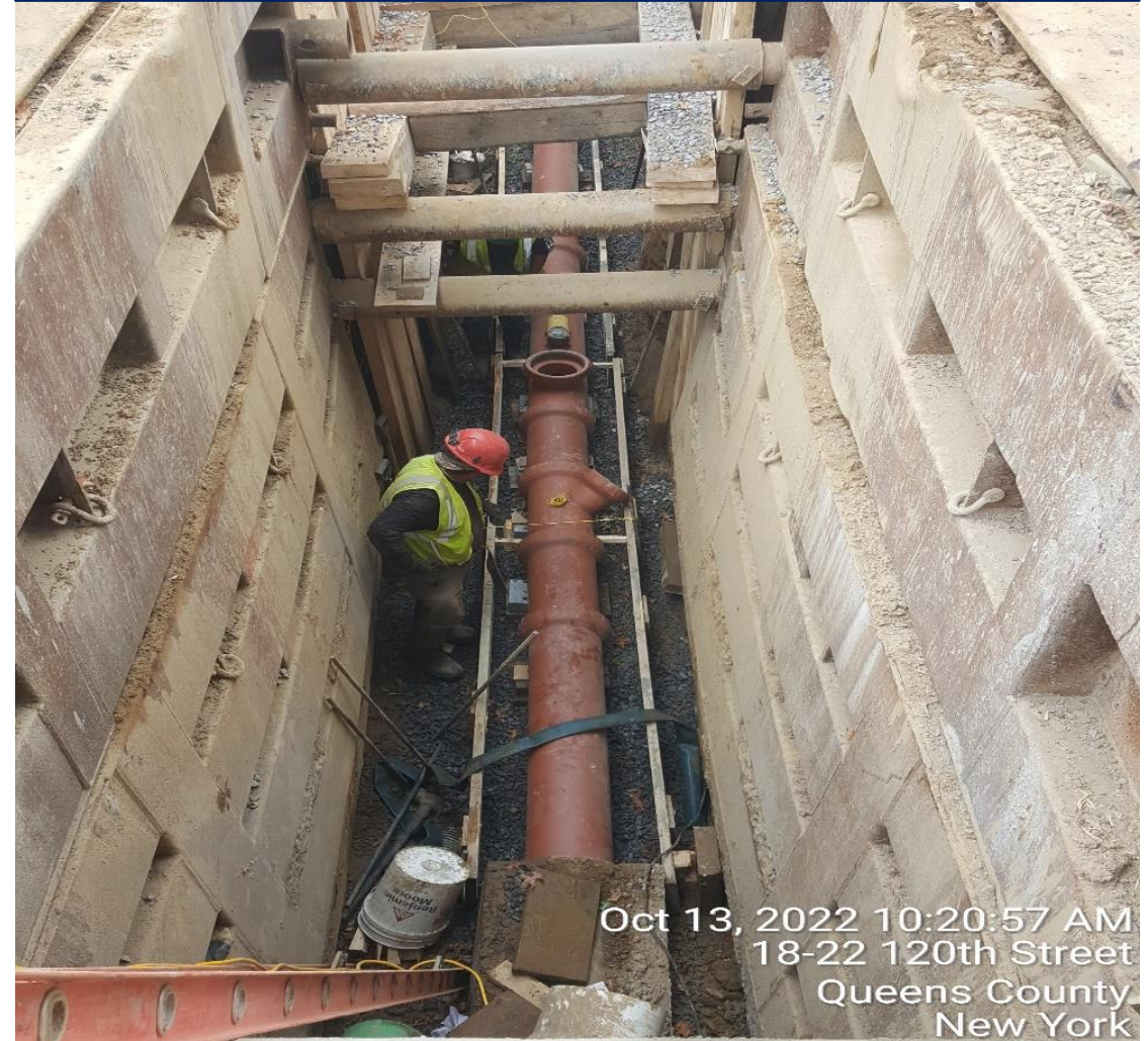
10" dia ESVP Sanitary Sewer 120 th Street between 20 th Avenue and 22 nd Avenue
