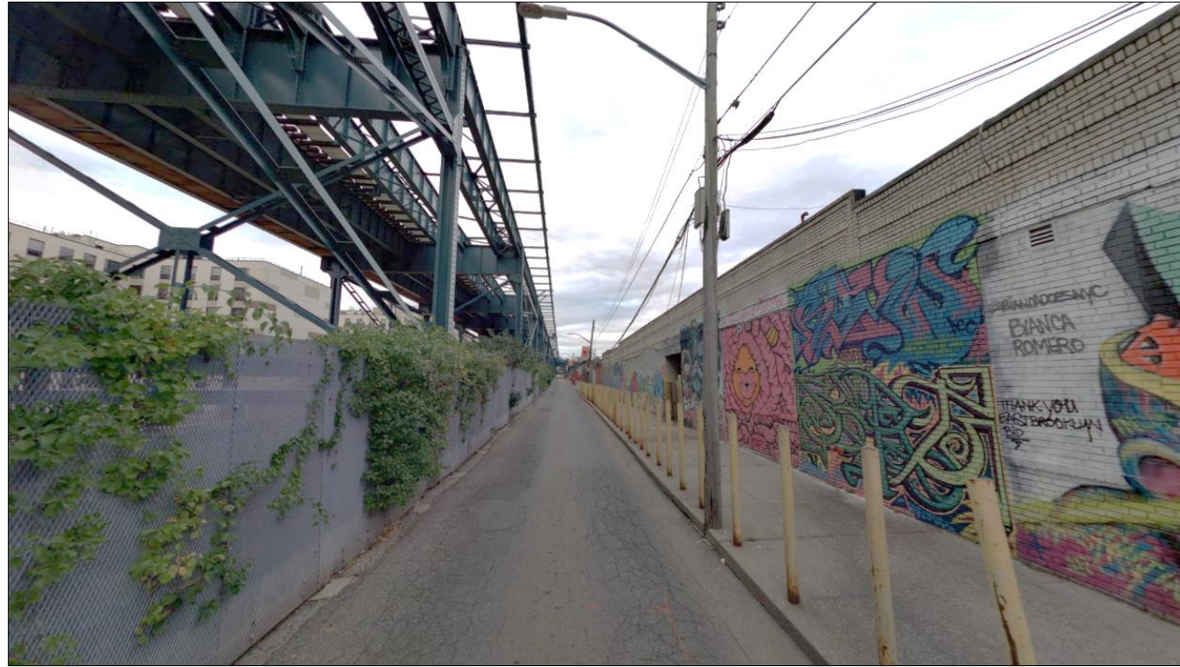
#3 Existing MTA fence, roadway condition, non-standard concrete sidewalk, and metal posts along Van Sinderen Avenue near Glenmore Avenue.
