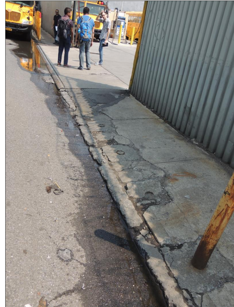
#4 Ponding and deterioration of sidewalk in front of the school bus parking lot near Pitkin Avenue Intersection.
