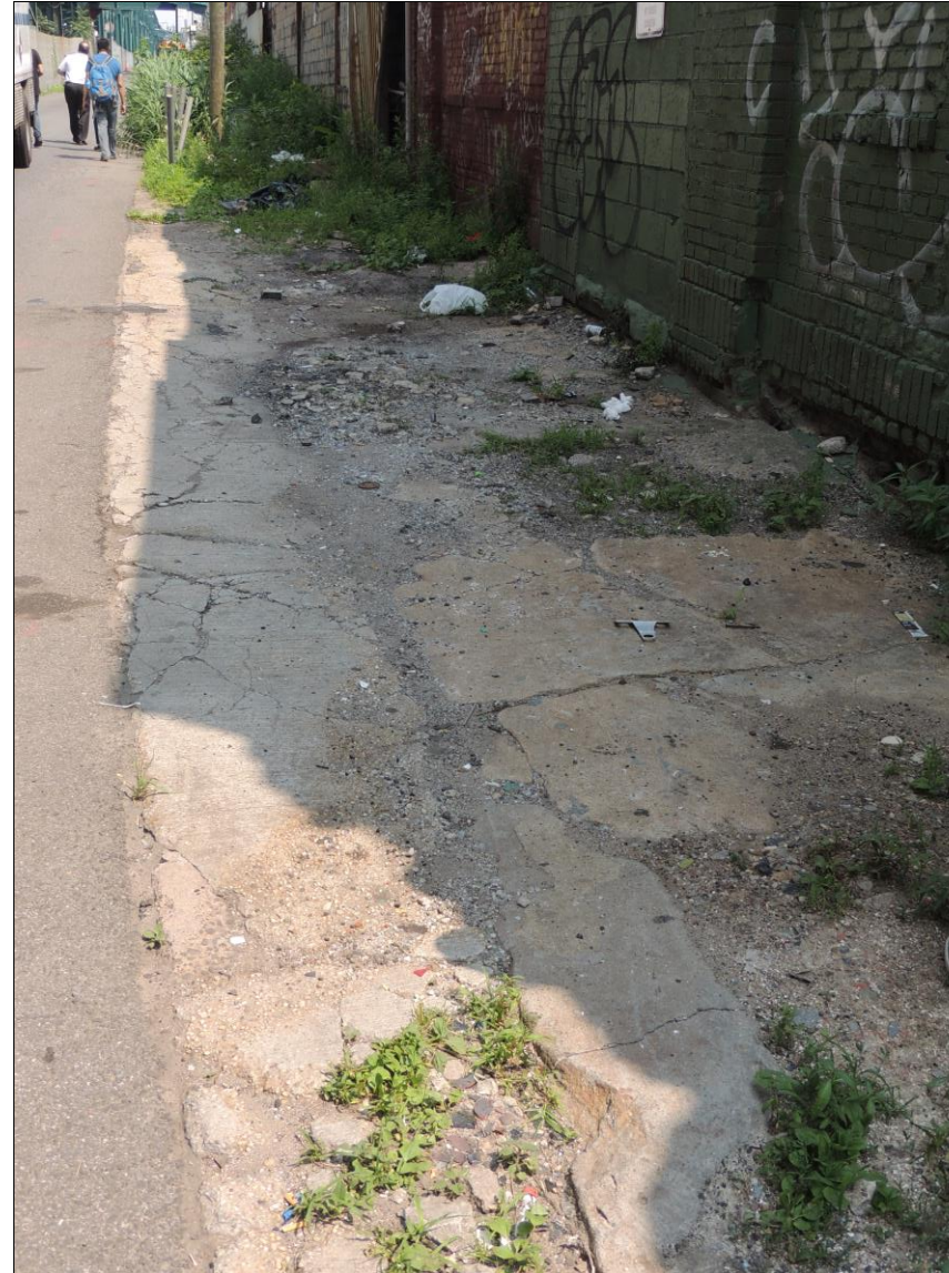
#6 Undesirable vegetation and broken sidewalk along Van Sinderen Avenue between Pitkin Avenue and Belmont Avenue.
