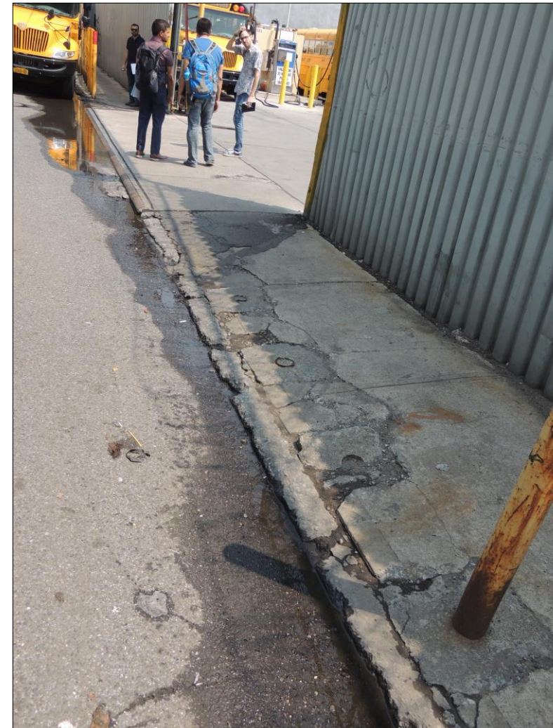
#4 Ponding and deterioration of sidewalk in front of the school bus parking lot near Pitkin Avenue Intersection.
