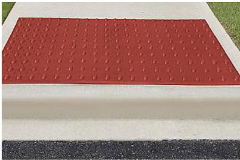
RED DETECTABLE WARNING STRIP
