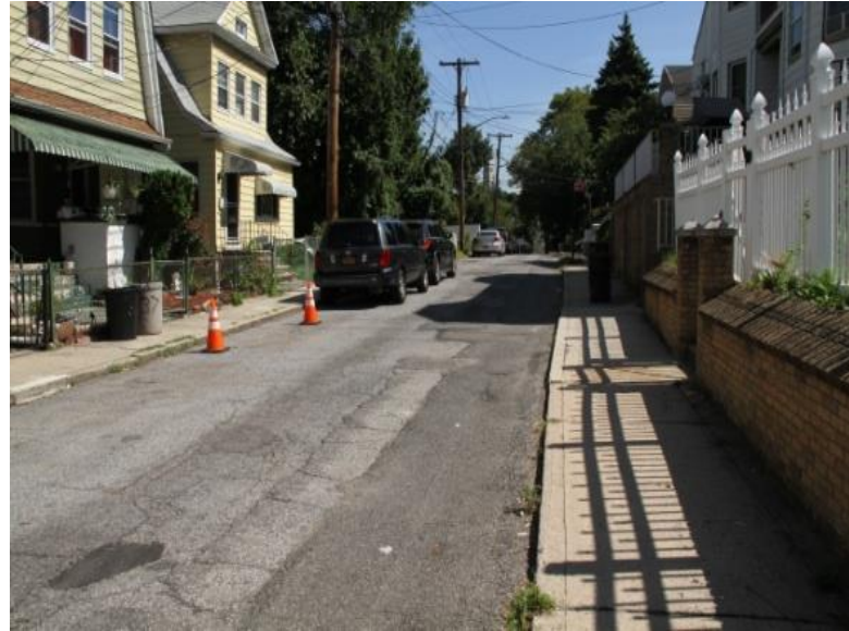
Picture 7: Existing Roadway and Southern Sidewalk I/F/O House No.40 (Photo taken looking towards York Avenue)
