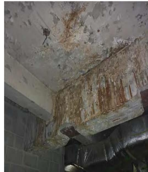
Concrete slab damage
