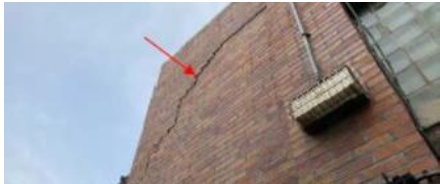
Diagonal and horizontal cracks in the masonry with no reinforcement.
