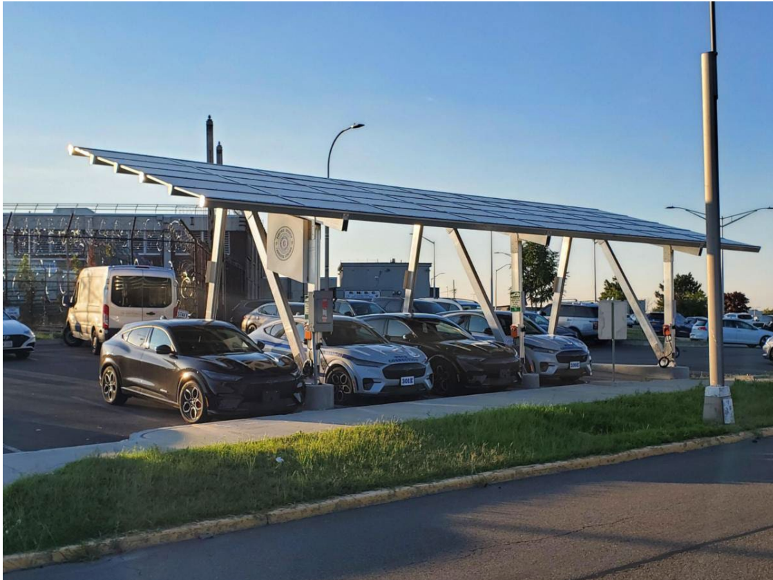
New Department of Correction Solar Canopy installed at Riker's Island.
