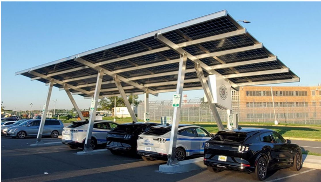
New Department of Correction Solar Canopy installed at Rikers Island
