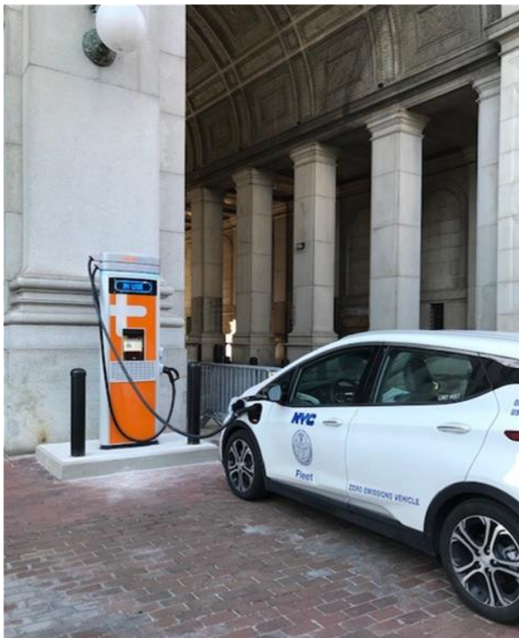
DCAS Fleet Chevy Bolt charging at one of the David N. Dinkins Manhattan Municipal Building's two fast chargers.
