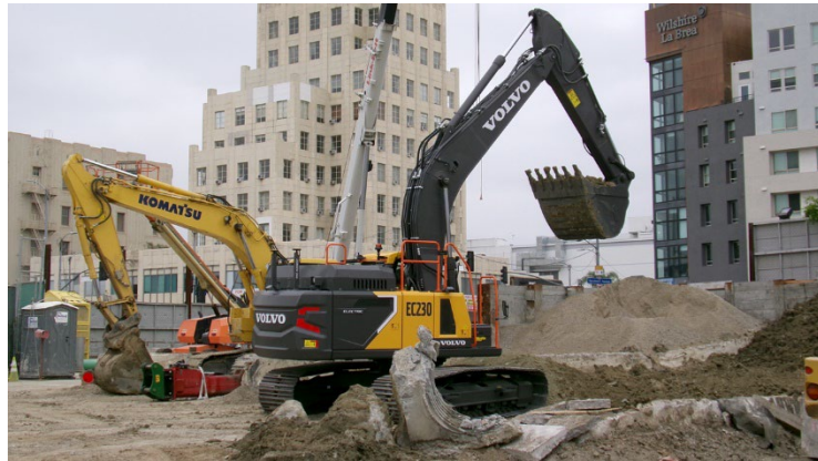
Figure 5. Volvo EC230 Excavator on site at the Los Angeles Metro Purple (D Line) Extension (2023)
