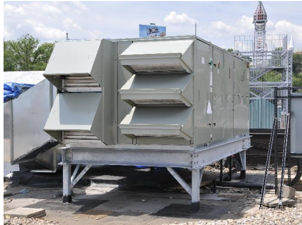
Upgraded rooftop unit
