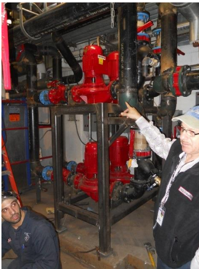
Chilled water pumps
