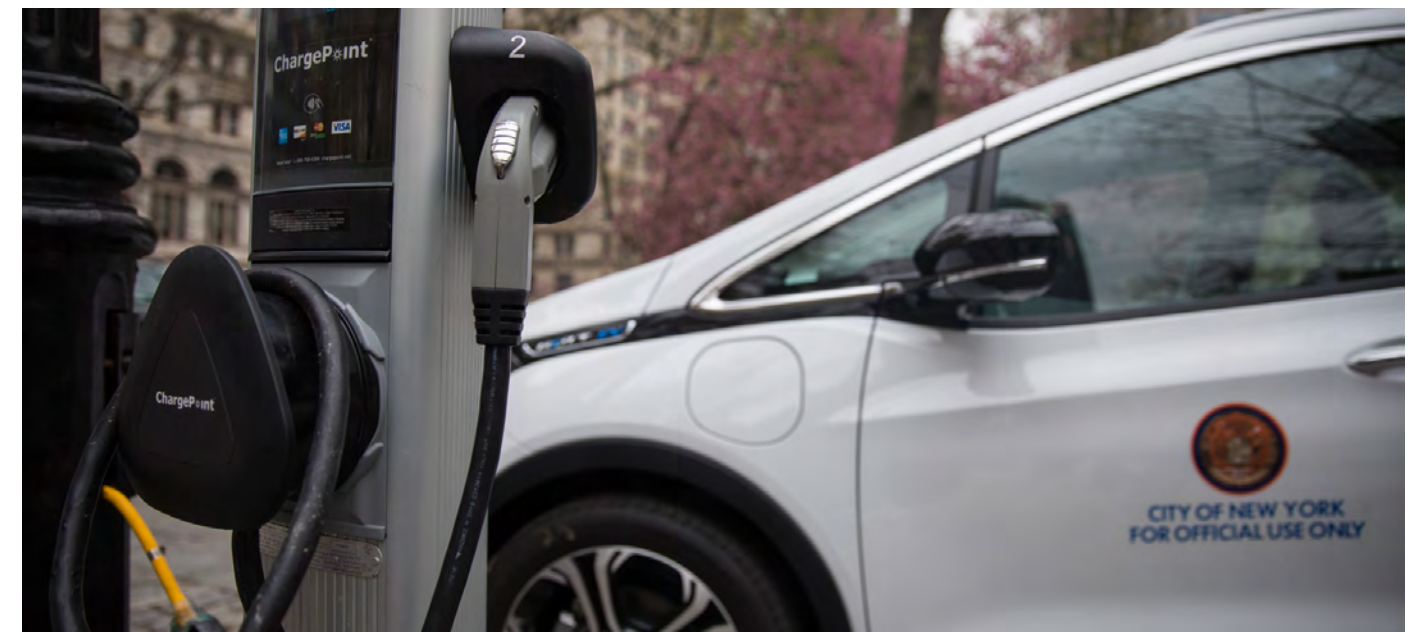
EV charging infrastructure for the NYC municipal fleet. Source: MOCEJ.
