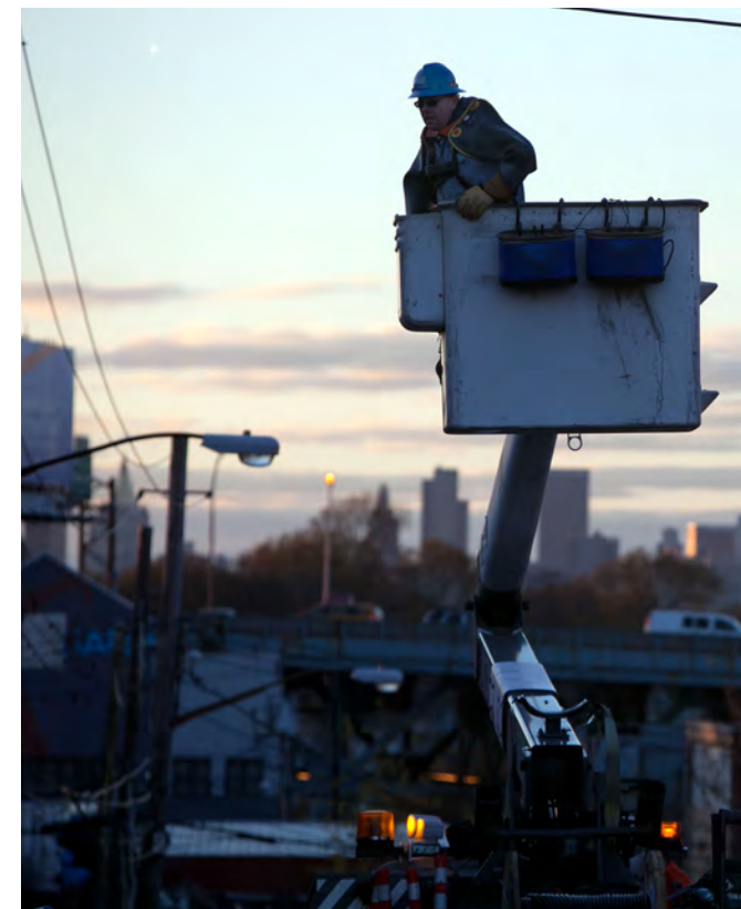
Utility hardening, Maspeth, Queens. Source: MOCEJ
