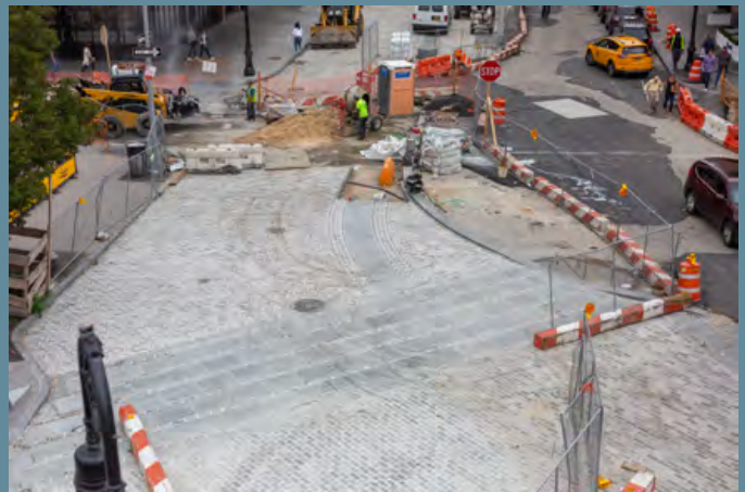
THE GANSEVOORT STREET AREA RECONSTRUCTION IN THE MEATPACKING DISTRICT OF MANHATTAN INCLUDES THE REPLACEMENT OF WATER MAINS AND CONSTRUCTION OF CATCH BASINS—IN ADDITION TO TREE PLANTING, PLAZA RECONSTRUCTION, AND DECORATIVE PAVING.
