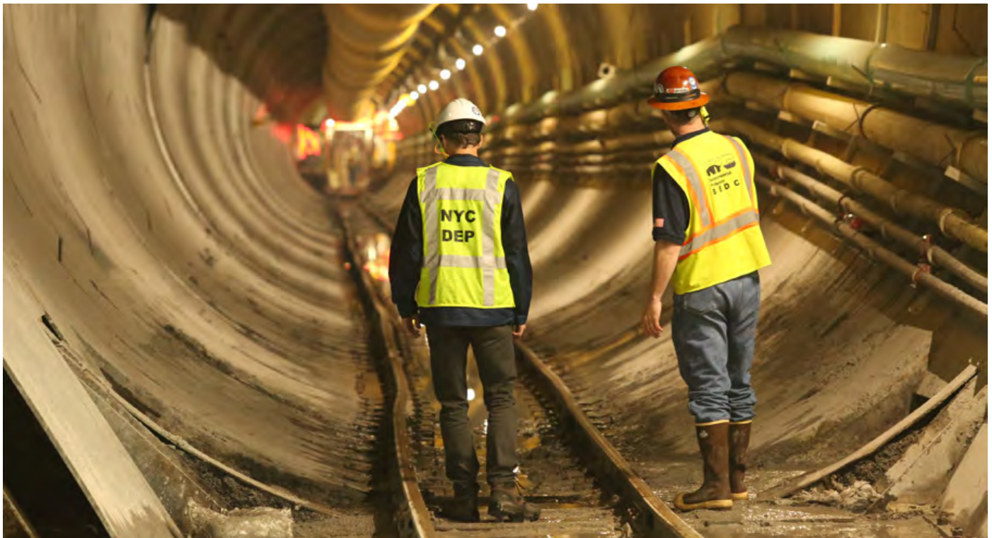
WORKERS IN THE DELAWARE AQUEDUCT BYPASS TUNNEL, WHICH WILL HELP ENSURE THE SAFETY, RELIABILITY, AND RESILIENCY OF THE CITY'S WATER SUPPLY.
