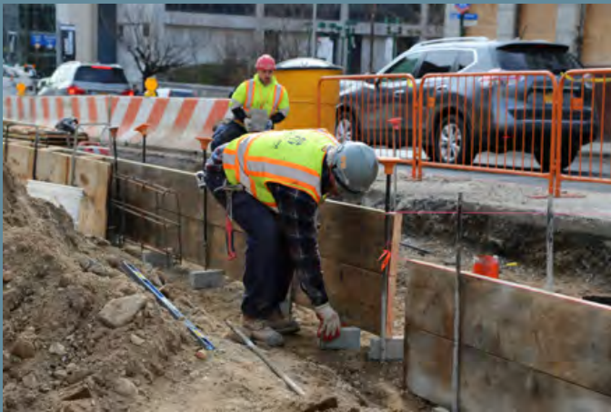
THE RECONSTRUCTION OF TILLARY STREET WILL CREATE A SAFER AND MORE WELCOMING GATEWAY TO BROOKLYN. THE PROJECT INCLUDES TRAFFIC SAFETY, LANDSCAPING, AND DESIGN IMPROVEMENTS AND WILL REPLACE MUCH OF THE UNDERGROUND INFRASTRUCTURE.
