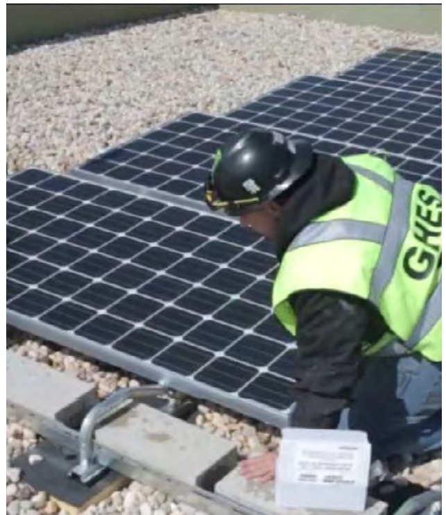
Solar installation in NYC
