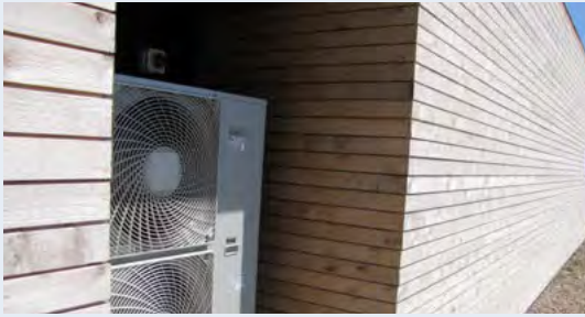
Residential heat pump installation
