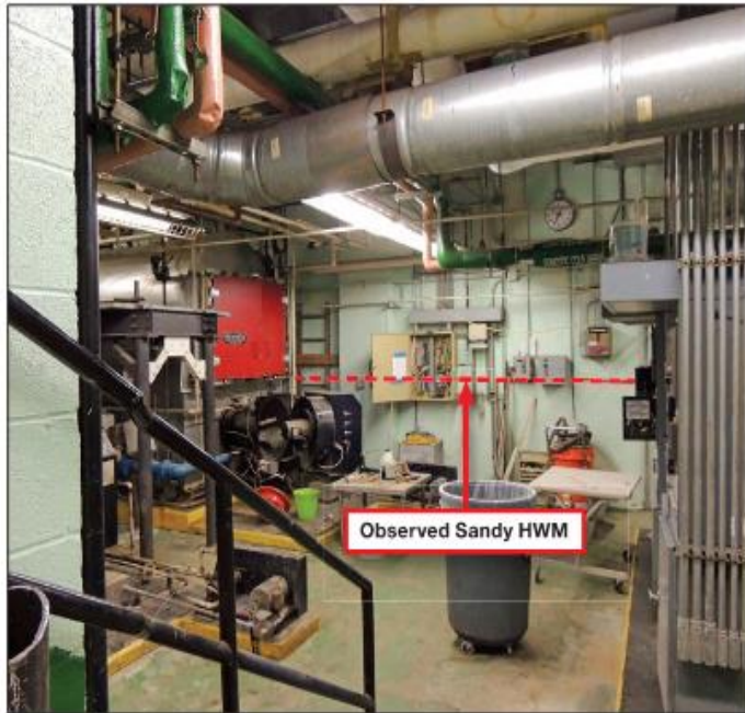
Figure 5-10: The basement of PS43 was inundated with approximately 5 feet of water (Queens, NY)
