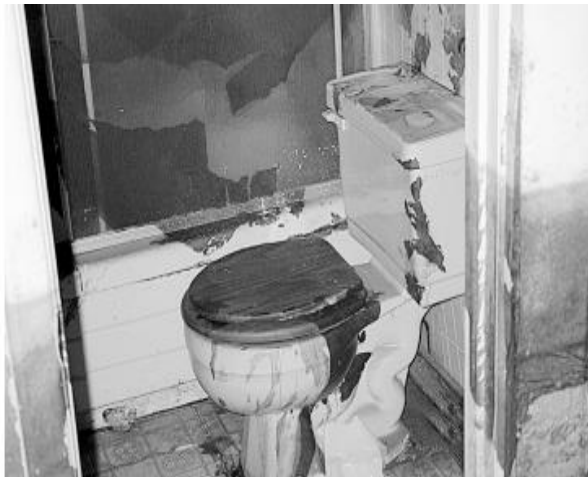
Figure 1.2.1D: The result of sewage back-up through a toilet during a riverine flooding event
