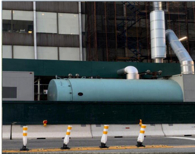
3. Temp. DOB registered oil-fired mobile boiler and fuel oil storage tank with associated piping at a site for emergency heating.
