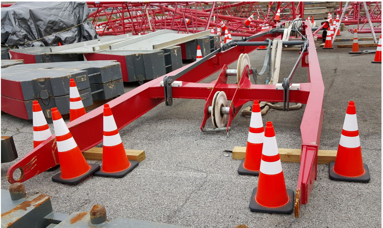
Photo 11 – A-frame disconnected from jib heel
