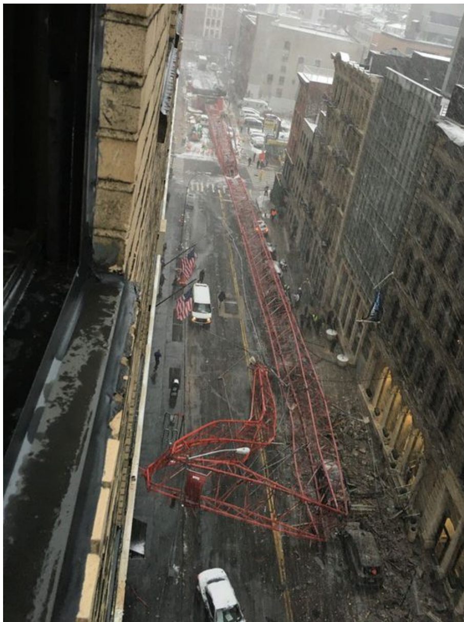
Figure 3 – Overturned crane lying along Worth Street, looking WNW [Ref. 15]
