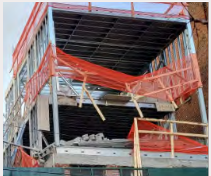
A knuckleboom deposited CMU block on a deck before the framing system was complete, overloading the deck.
