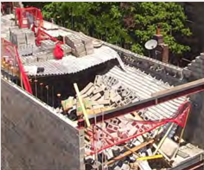
CMU blocks were stacked on a deck supported by cold-formed joists without adequate shoring, overloading the deck.
