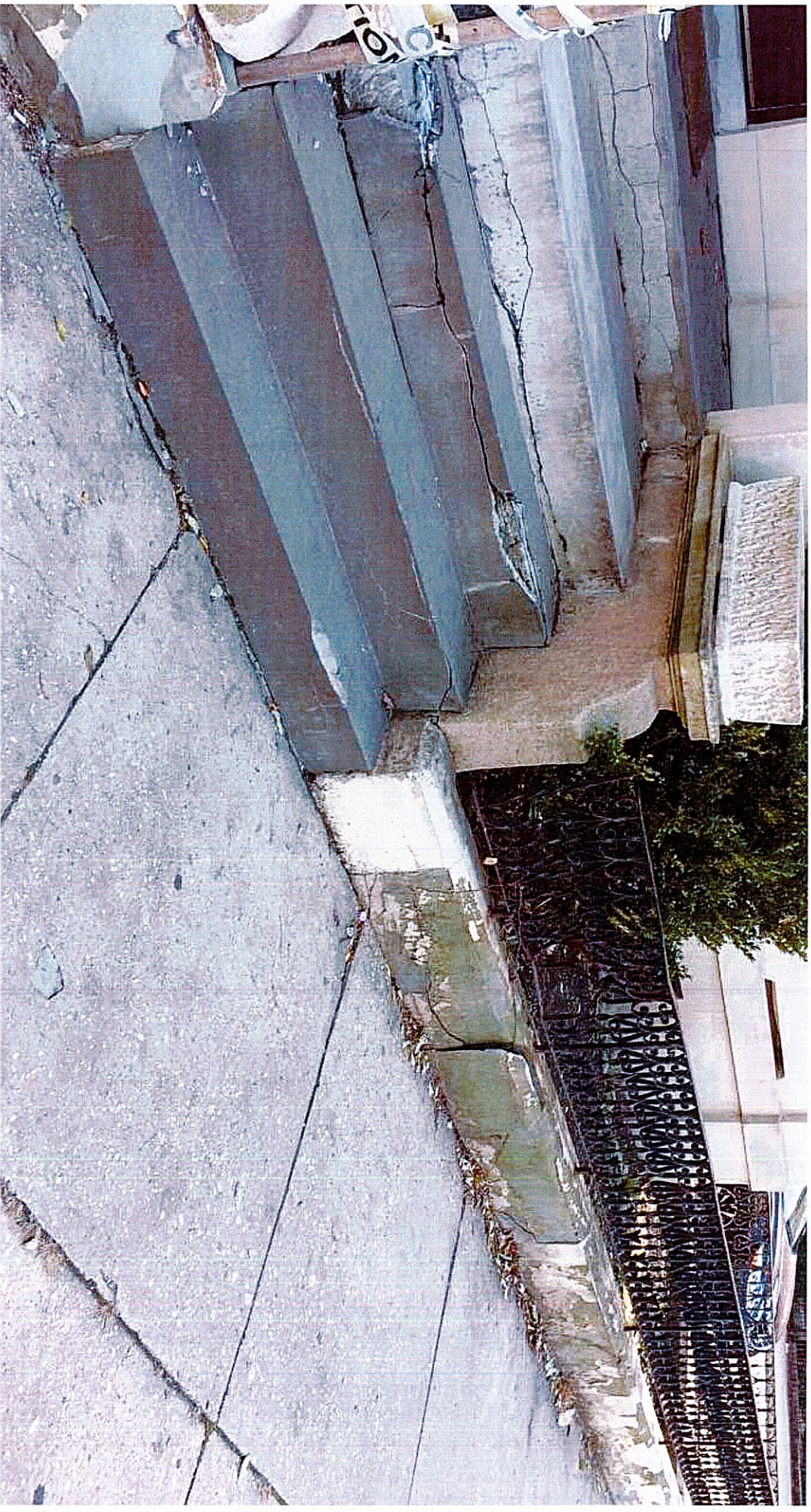
Photo illustrating the condition of the curb, low railing, and Rutland Road Entry Stair after the accident of January 23rd, 2017
