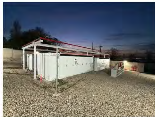
NineDot Energy Battery Energy Storage Site in New York City
