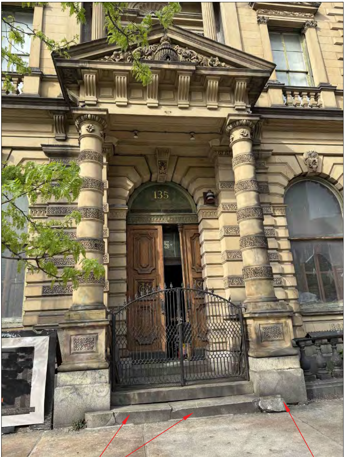
REMOVE EXISTING BROKEN STONE STEP AND REPLACE WITH NEW SOLID STONE (GRANITE) STEP
