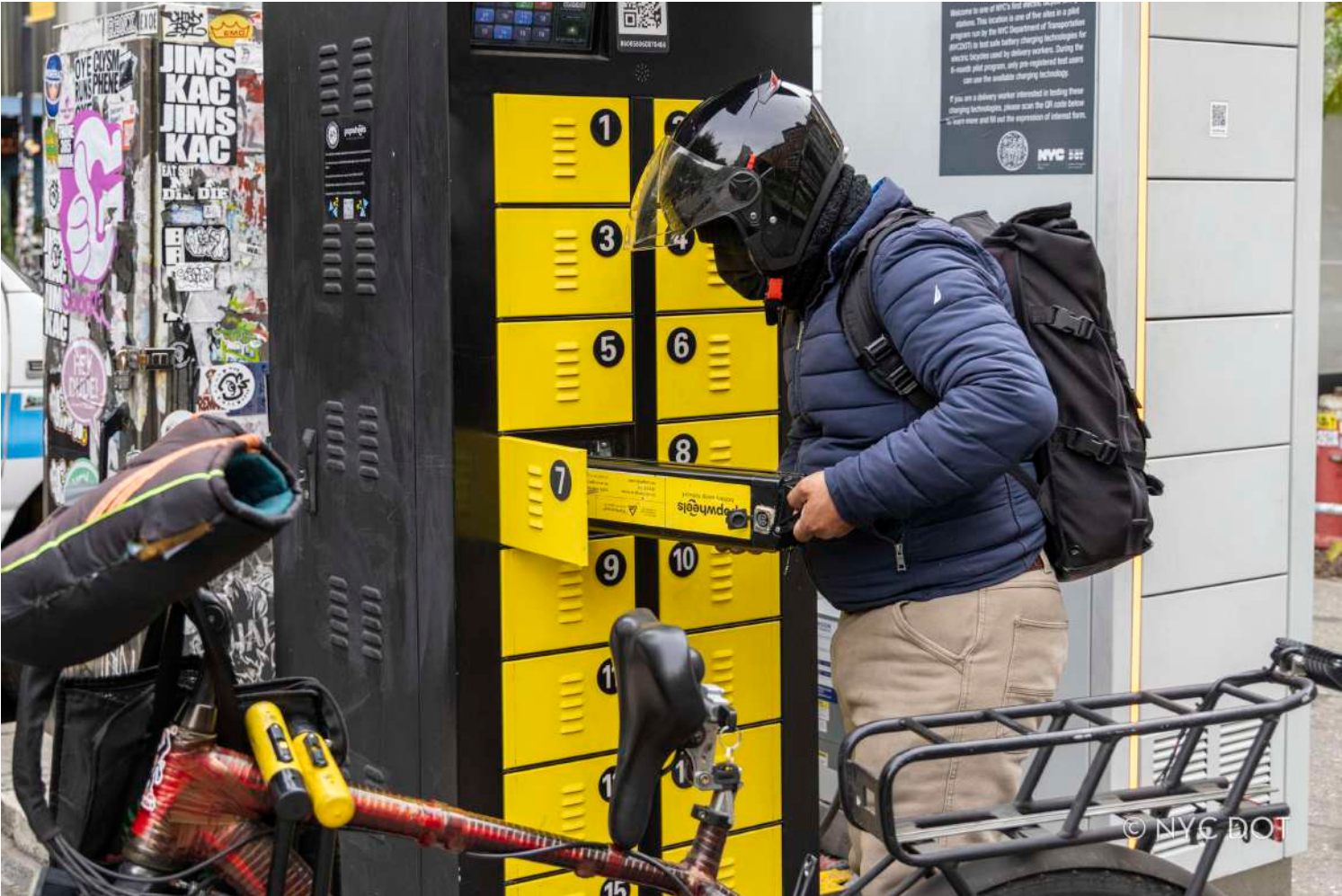
During the E-Bike Battery Charging Pilot in 2024, e-bike riders tested e-bike battery-swapping cabinet technology located on public sidewalks.
