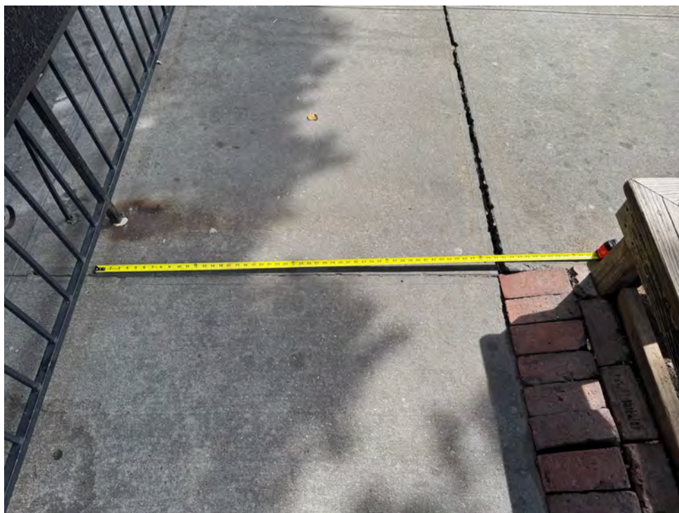
Only 4 feet of sidewalk on Oak Street
