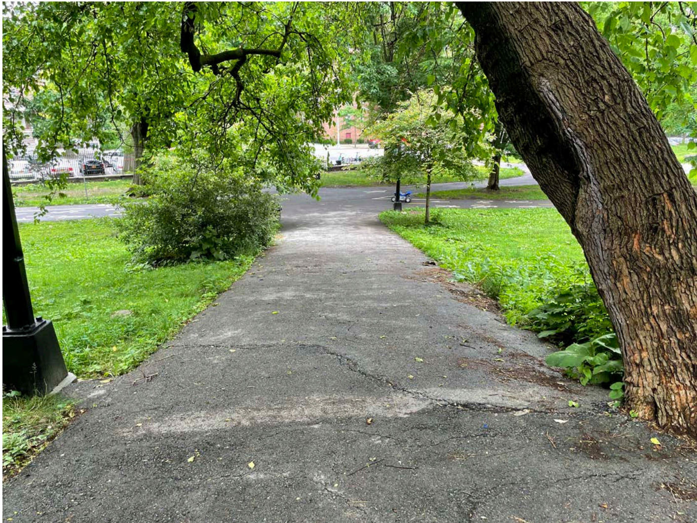
1 - midway down ramp, showing encroaching tree and bottom of ramp
