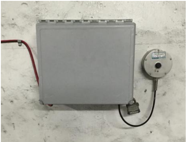
Typical Indoor Seismograph Installation
