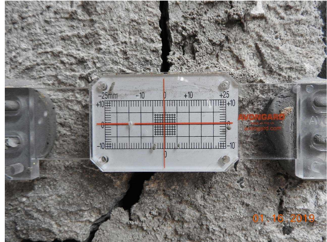
Typical Representation of a Crack Gauge
