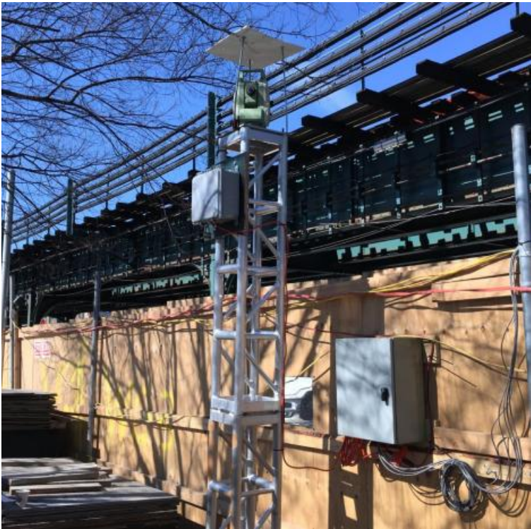
Typical ATMS Pedestal Installation
