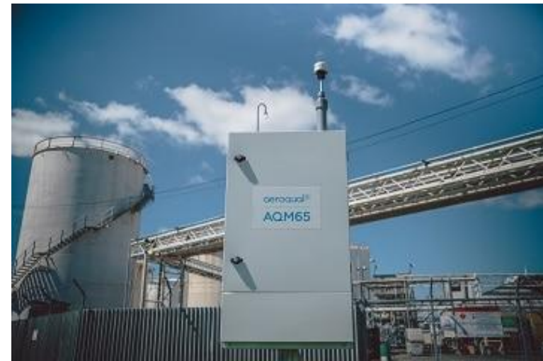
Example of Air Monitoring Station (Not Bronx Project)
