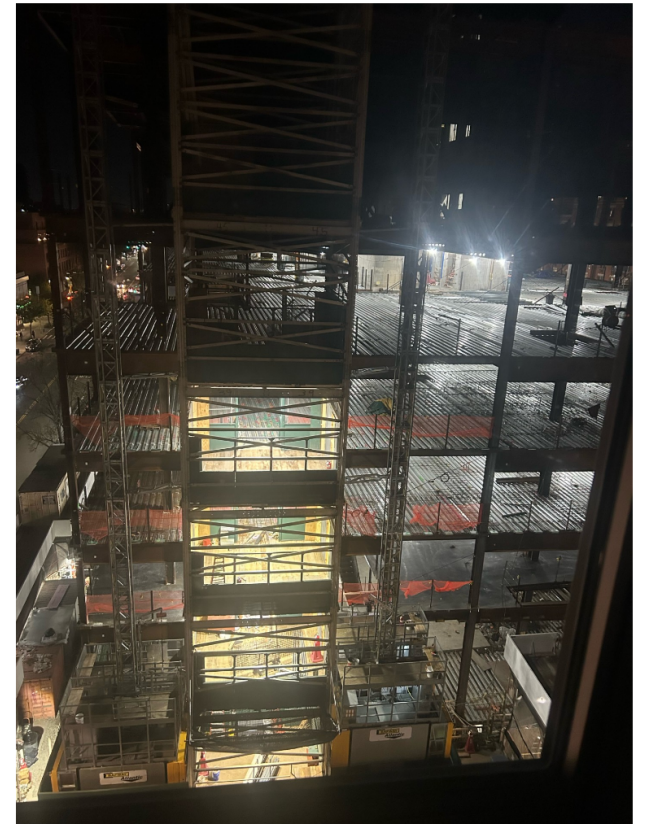
Smith Street Hoist Landings
