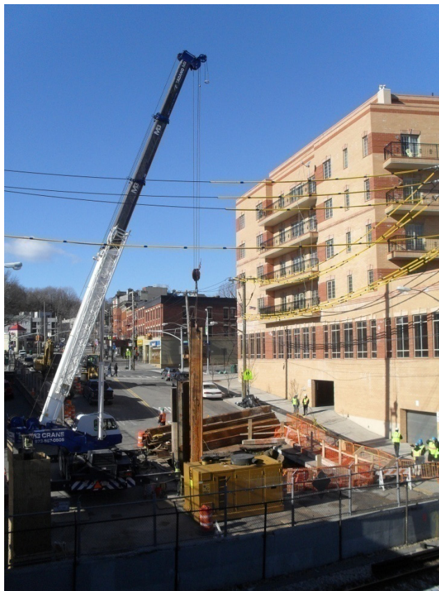
Installation of sheeting for jacking pit, Victory Boulevard just west of SIRR tracks (looking west towards Bay Street)
