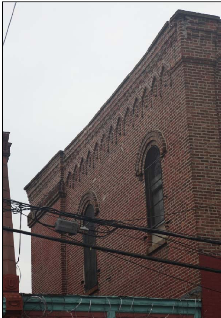
William Ulmer Brewery Engine and Machine House, Southwest Facade Photo: Christopher D, Brazee, 2009
