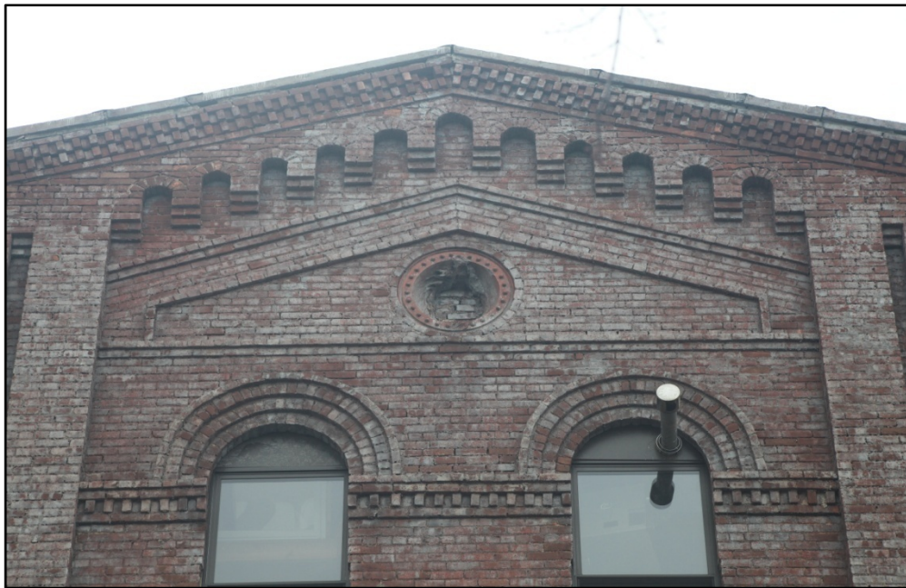
William Ulmer Brewery Stable and Storage Building, Cornice Detail Photo: Christopher D. Brazee, 2009
