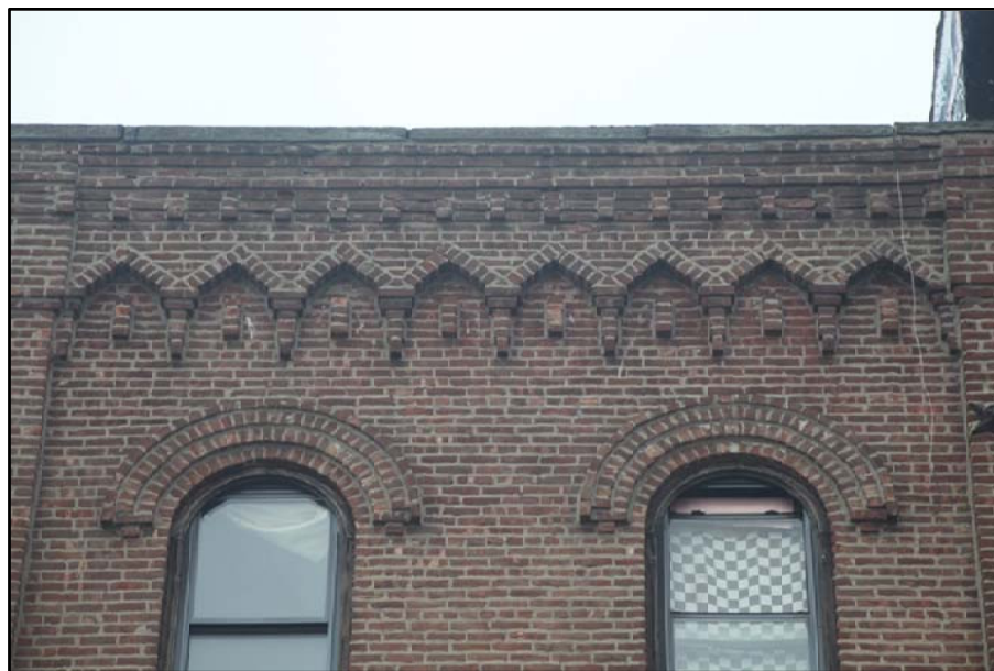
William Ulmer Brewery Engine and Machine House, Cornice Detail Photo: Christopher D, Brazee, 2009
