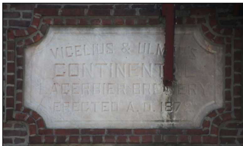
William Ulmer Brewery Main Brew House, Date Stone Detail Photo: Christopher D. Brazee, 2010
