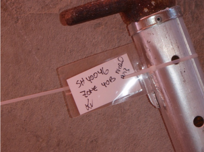
Photo 4 Typical Tag and Failure at Connection Note Name, Zone and Signature
