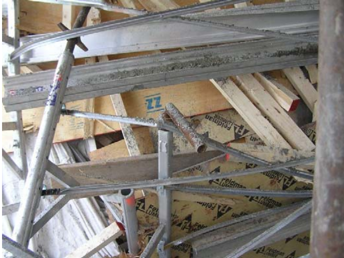
Photo 26 Broken Adjustment Screw Extension
