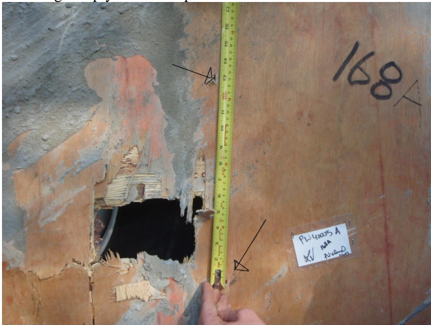
Photo 21 Plywood Penetrated by Leg Base
