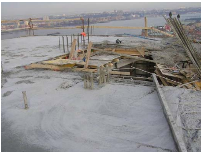
Photo 3 42nd Fl. Debris - Looking North East
