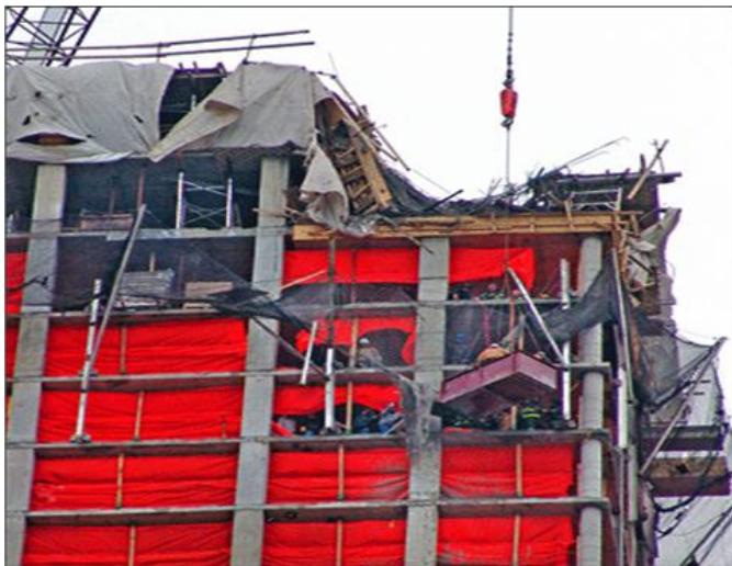
Photo 1 Collapse Area - Looking West
