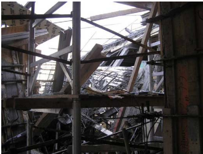
Photo 2 Debris Field 41st fl.
