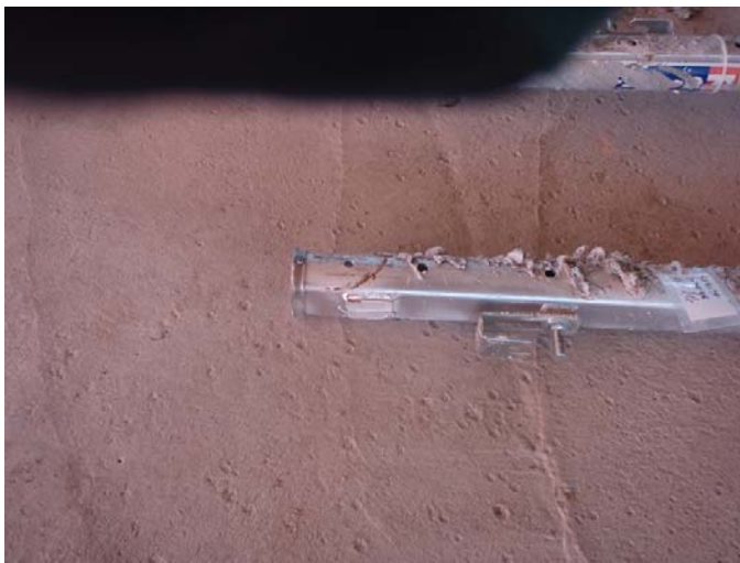
Photo 10 Fracture near Weld
