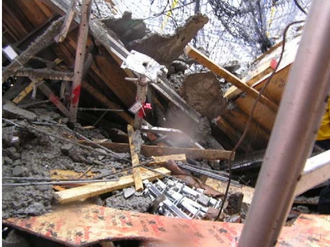
Photo 9 Bent Top Plate
