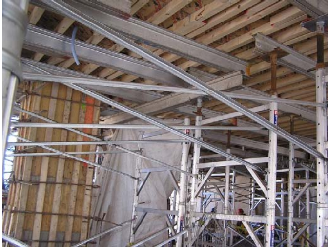
Photo 15 Improper Stringer Setting
