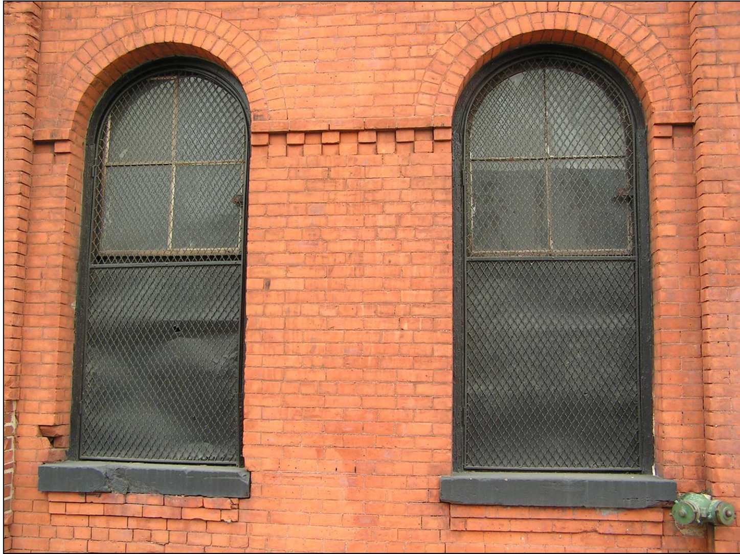
Estey Piano Company Factory, first-floor windows on Lincoln Avenue façade. Photo: Michael Caratzas
