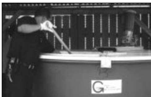
Jamaica Market staff add fruit and vegetable scraps to one of the Market's composters. Composting equipment is installed in a protected area behind the Market.
