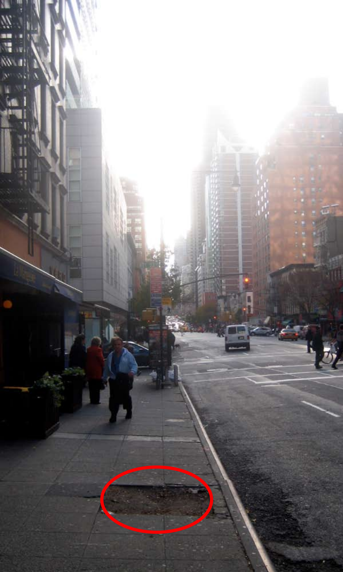
Near Vero Wine Bar there are missing street trees with the tree well still exposed creating a set of hazardous conditions on the sidewalk for pedestrians as well as an unpleasant streetscape.
