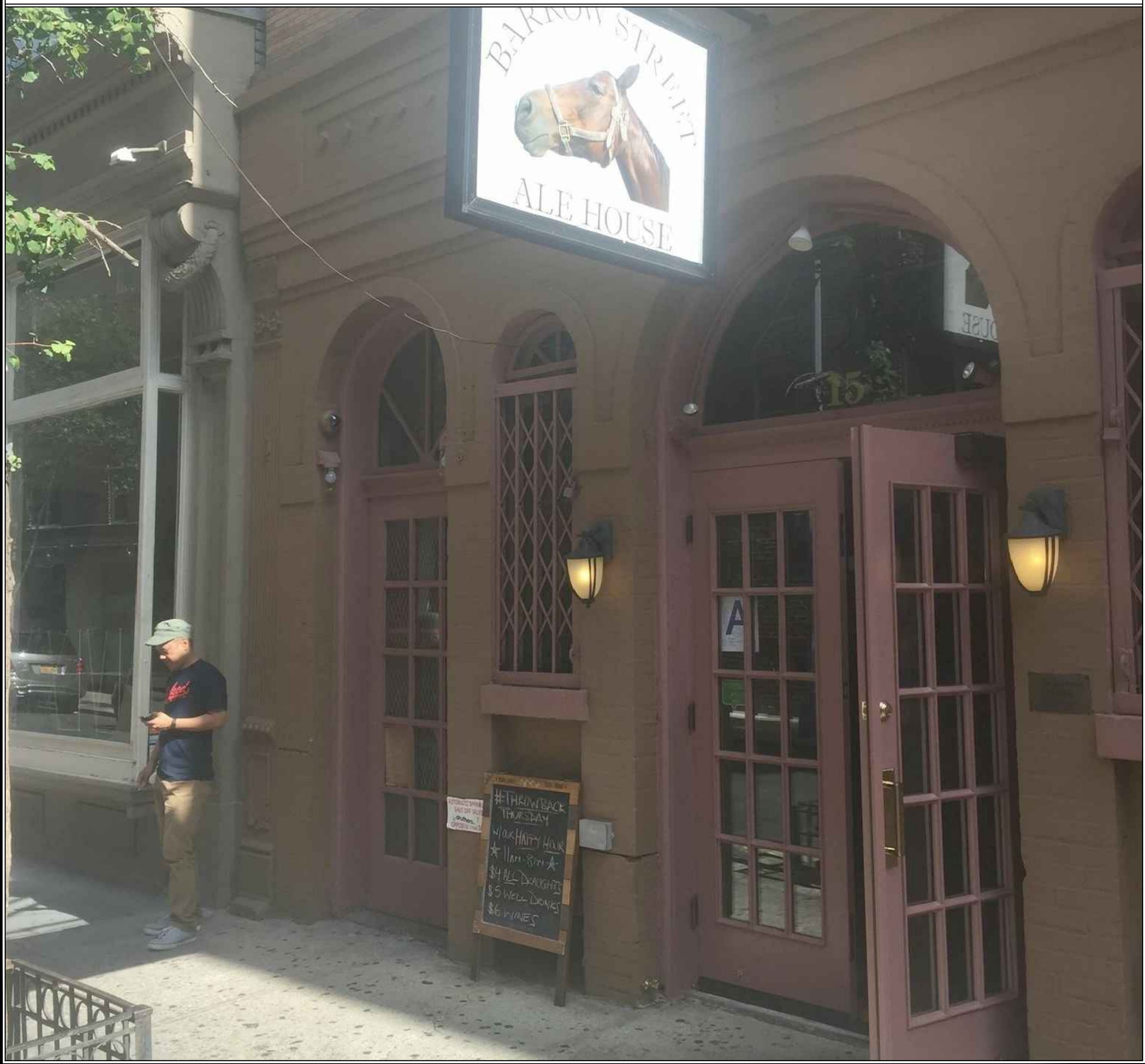
EXISTING FACADE CONDITIONS
