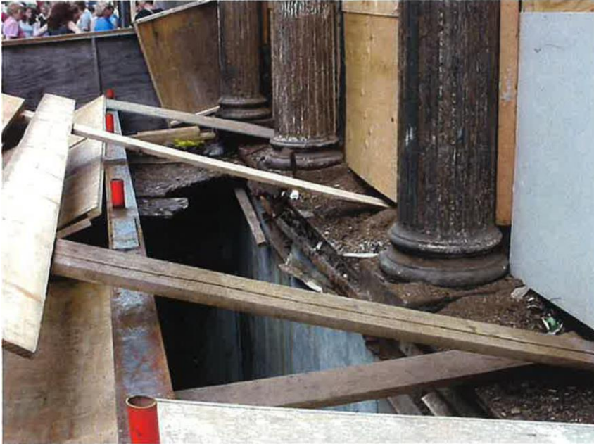
STREET VIEW: SIDEWALK VAULT – AFTER COLLAPSE IN JULY 2001 – NOTE DAMAGED LIGHTS AND STEPS
