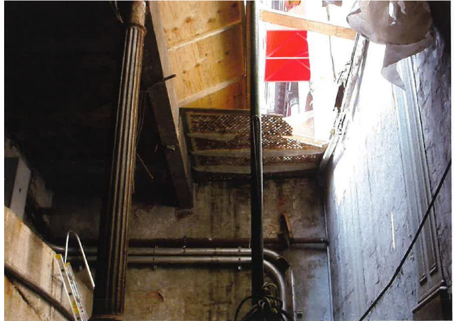
VAULT VIEW: SIDEWALK VAULT AFTER COLLAPSE IN JULY 2001 – NOTE DAMAGED LIGHTS
