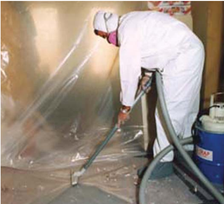
A lead abatement technician cleans up a contaminated site using a special wet vacuum.
