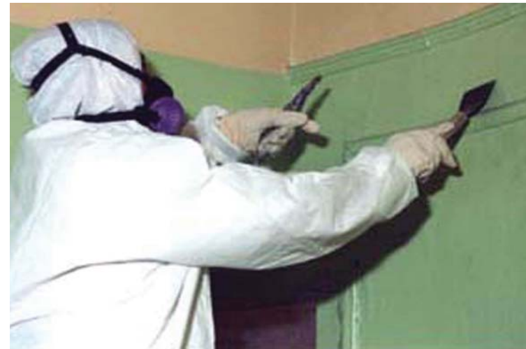
An abatement technician with appropriate protective gear removes paint from a wall.
