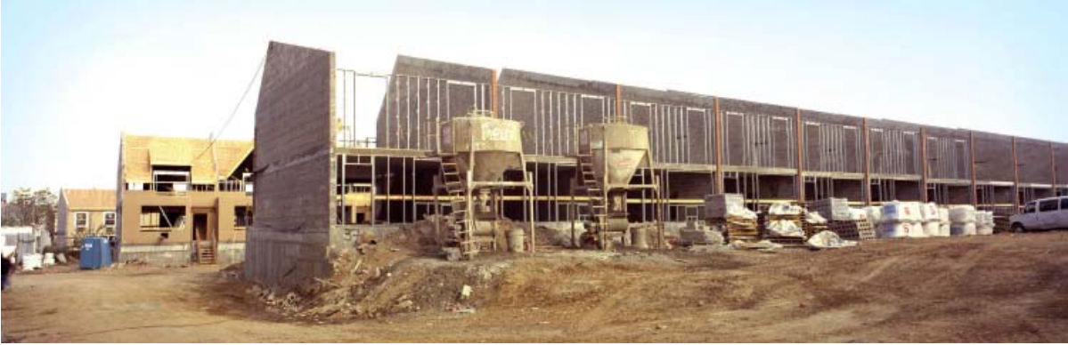
Formerly the site of the Rheingold Brewery, this is the first comprehensive redevelopment of a City-owned brownfield site. It is a planned result of an international design workshop undertaken with active involvement from the community, government agencies, and the International Brownfields Exchange. Approximately 250 apartments and homes are currently in development.
