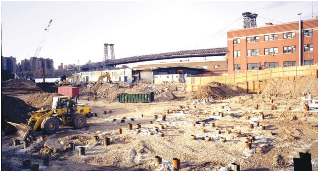
The former site of the Schaefer Brewery in Williamsburg, Brooklyn, under construction.
