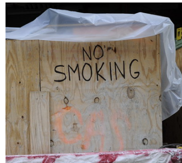
Unacceptable Warning Sign
