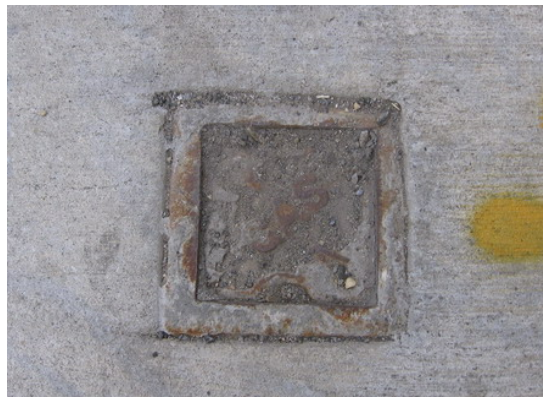
Gas shut-off valve in sidewalk
