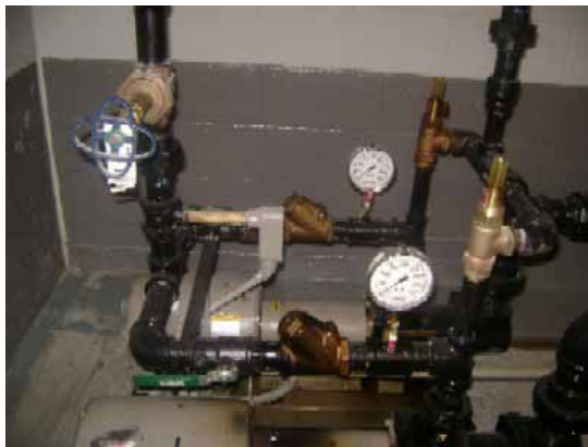
Pump connected to piping with the pressure gauge and control valves
