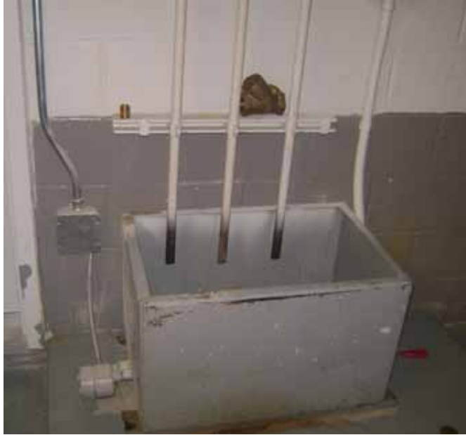
“Overflow catch Basin” or Tank with attached leak detection alarm
