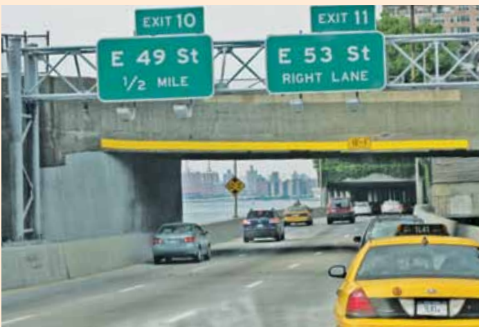
Bridge strikes at the E. 60 th / 61 st Street overpass on the FDR Drive are down 56% since the treatment was installed, the greatest reduction of any pilot location.
