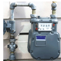
Gas meter with regulator and vent
